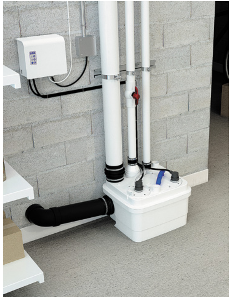
Installation above ground
