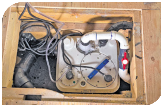
The Sanicubic 1 positioned in a small space under the floating home's wooden floorboard. AR Plumbing owner and CEO Adolfo Rodas and his team used two of the four inlets on the Sanicubic 1.
