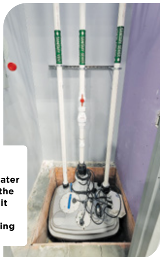
Sanicubic 2VX was installed in a closet that was created specifically for the pump on the other side of the bathroom.
